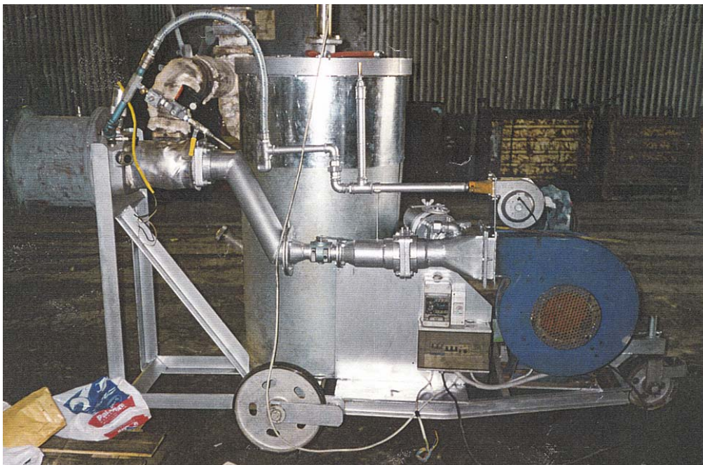
Photo 1: Picture of one of the downdraft gasifiers
